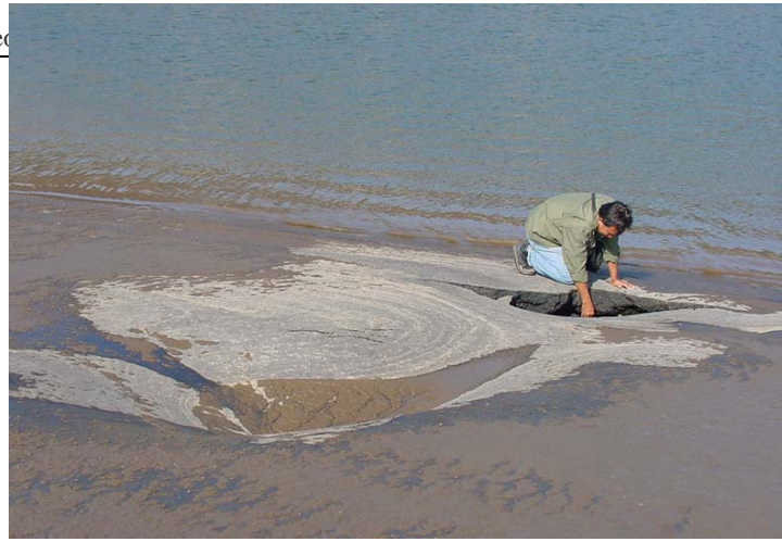
Fig.6 Rupture of asphalt lining on pond floor due to piping of leveling material underneath
